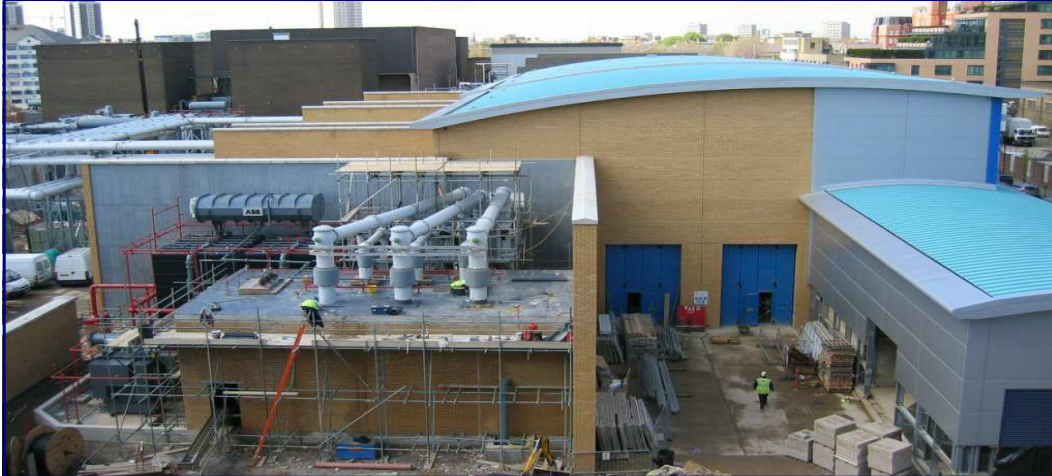
Super Grid Transformer Pens
