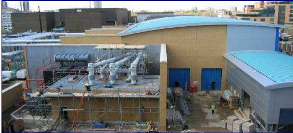
Super Grid Transformer Pens
