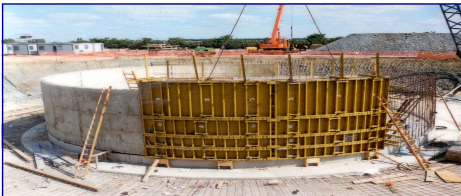
New Sewage Effluent Treatment Works
